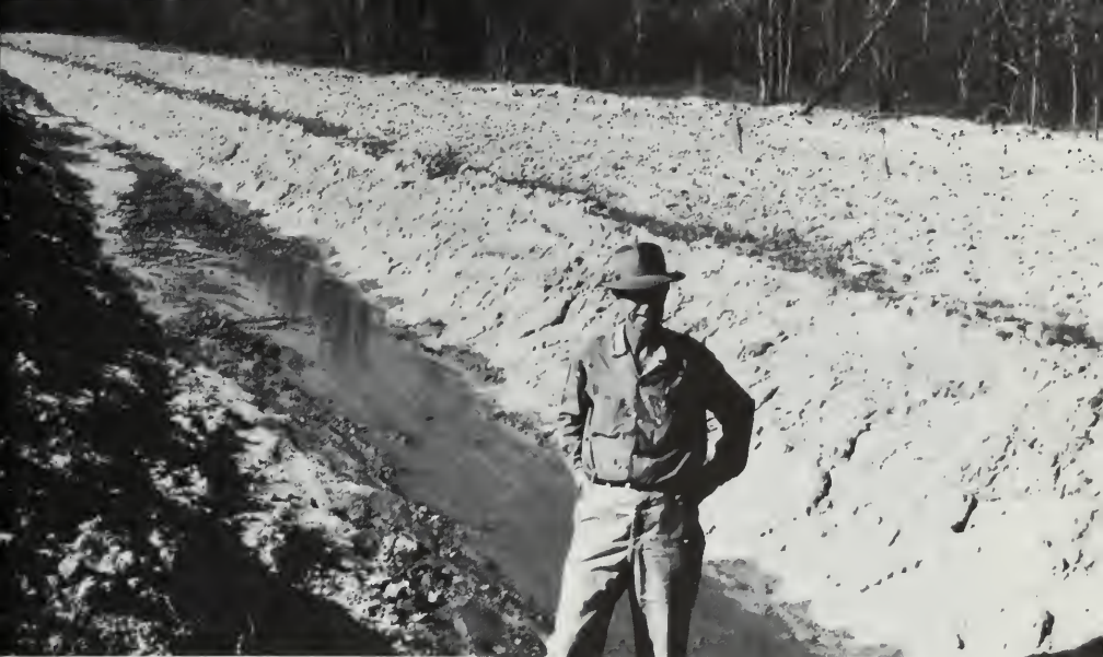
Soil Conservation Service technicians helped a farmer construct this drainage ditch in Logan County.
